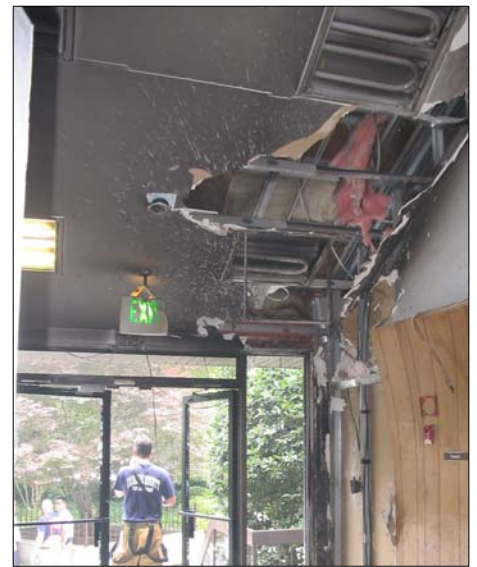
Damage to the front lobby of the building.
