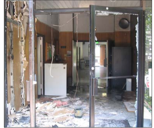
Damage to the front of the building.
